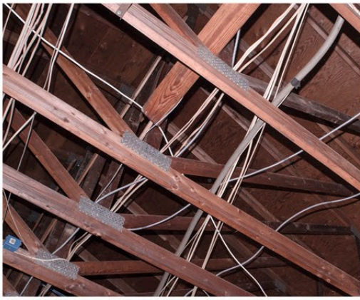
Exposed Ceiling Joists. Connect all wiring for housing before ceiling installation.
